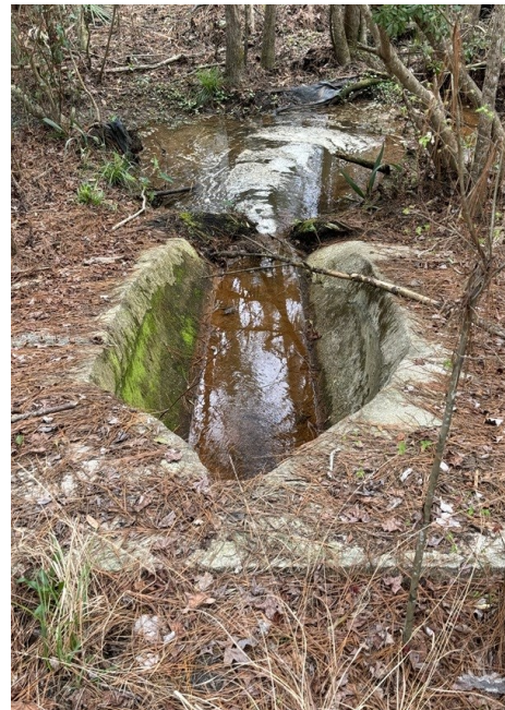
CONCRETE OUTFALL BY ARCH DAM (POND 5) WITH WATER DRAINING INTO SEATON CREEK
